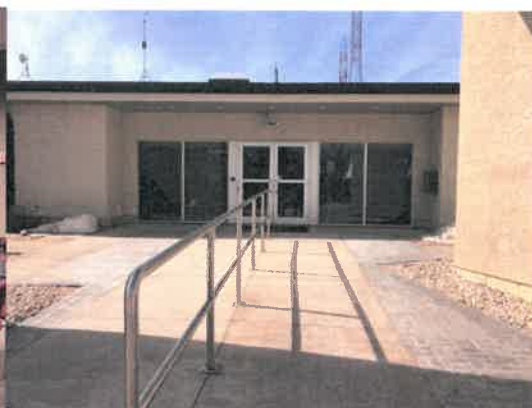
Front Entrance – Power assist doors & ramp with railing
